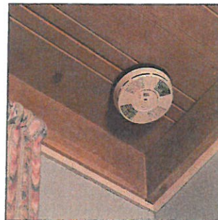
Smoke Alarm Monitor (71-108)
